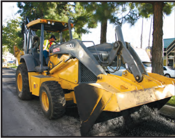
(Above) T.E. Roberts Construction Inc. installing a 13,000-foot recycle water main in El Monte, California for the Upper San Gabriel Valley Water District.
